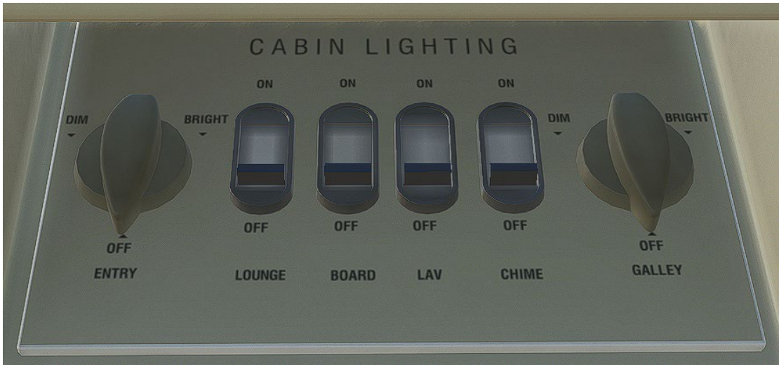
Figure 20-8 Cabin Lighting Panel — Forward Galley
